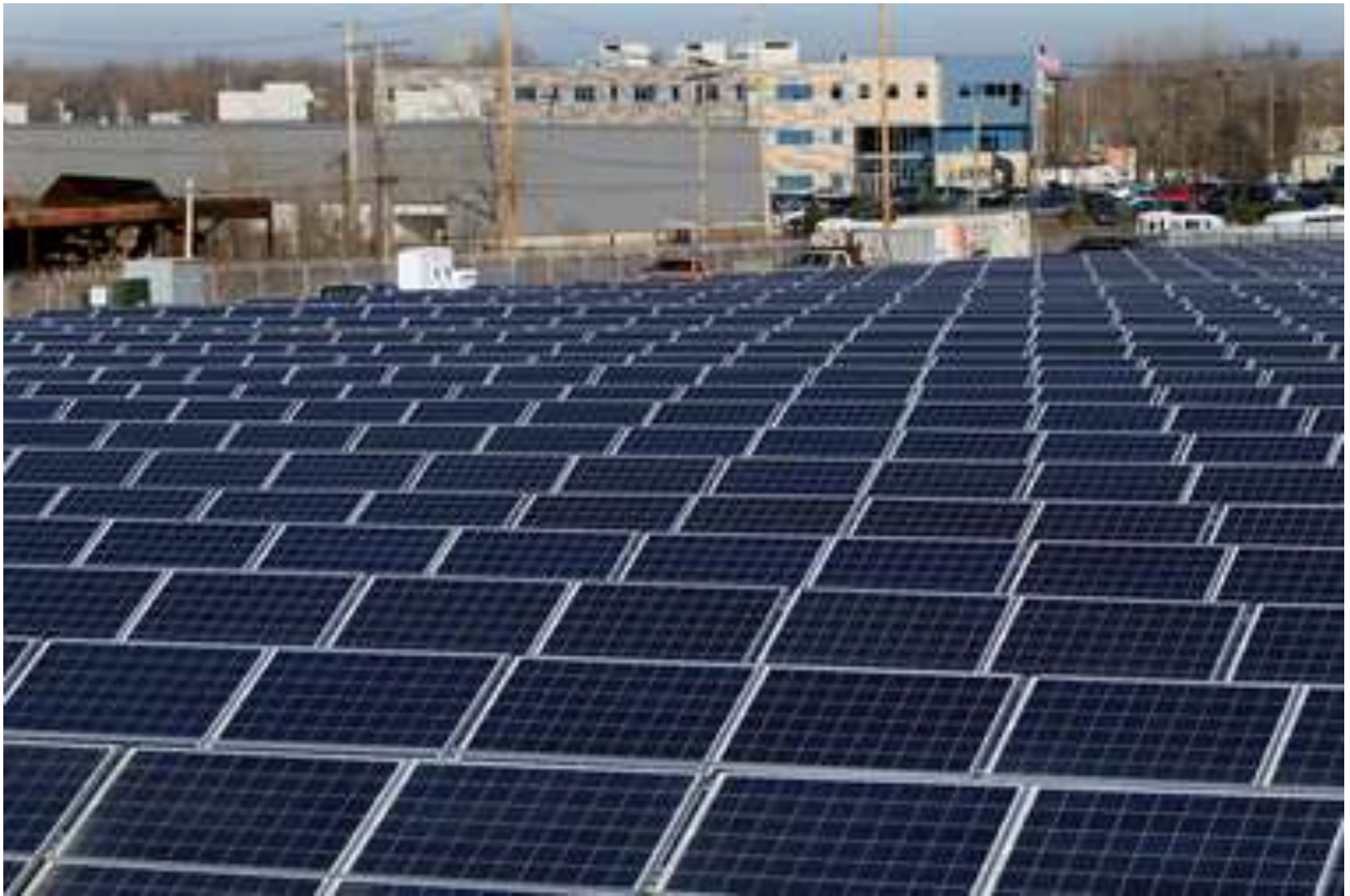
A six-acre solar farm occupies a former brownfield adjacent to the Cuyahoga Metropolitan Housing Authority headquarters on Kinsman Road in Cleveland
